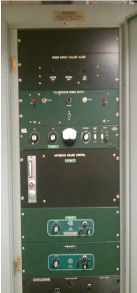
Station PA System
